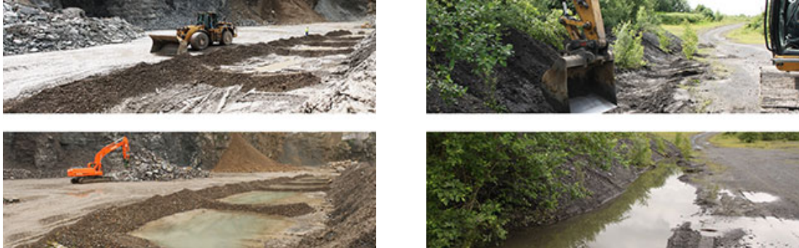
Figure 3: Channelling of running water in a multi-compartment basin at Lustin (Sagrex). Digging of a new ditch to collect running water on quarry tracks at Carrières du Hainaut.
